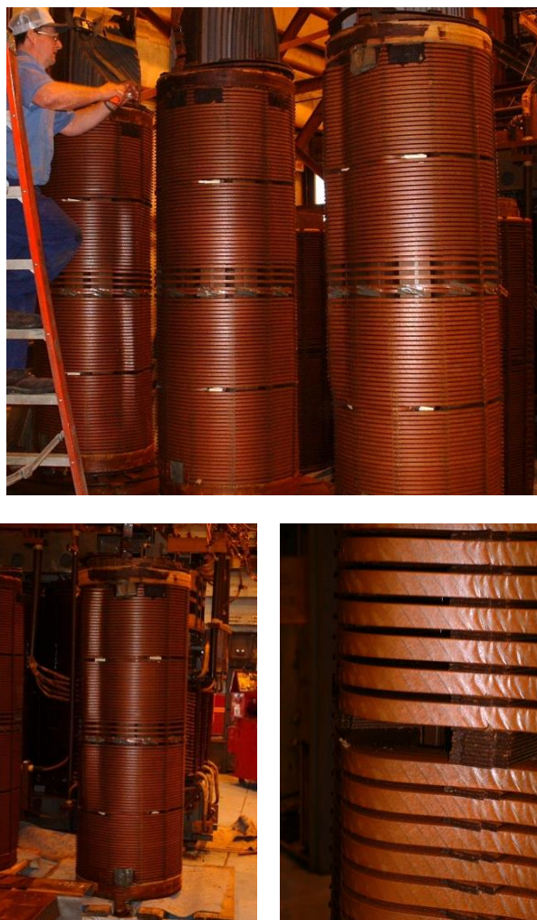
Figure 7: All three LV windings showing radial deformation (hoop buckling) and close up on phase C
